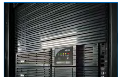
Simple steps like installing blanking panels in unused rack spaces can help prevent warm air from recirculating and improve cooling efficiency.
