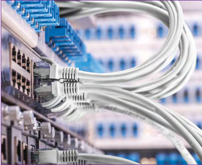
Cat8 cables make high-speed connections between 40 Gb switches, servers and other network equipment.
